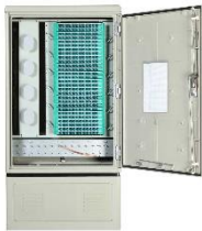
fiber cross connection cabinet
